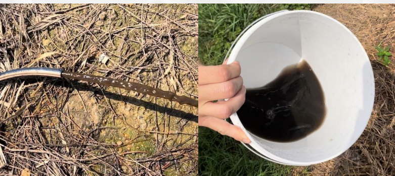
Figure 2. Water line flush after 12 hours of contact time of ProMax ® inside the water lines, showing the dark, smelly biogunk flushed from the scaled broiler drinker lines. ProMax ® was metered into the lines at 1:128 using a simple medicator pump.
