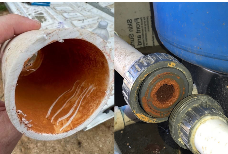
Figure 1. (Left) Iron scale hard film inside a brand-new (three-month-old) farm poultry water plumbing system; and (Right) water restriction at a pressure tank inlet on a broiler breeder farm, showing impact of iron bioscale on interior pipe diameter.
